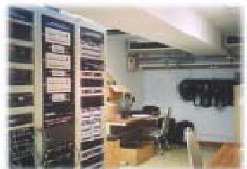
All equipment mounted on rack in control room
