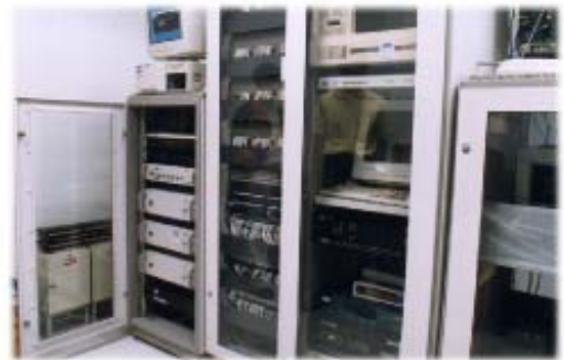
All equipment mounted on rack in control room
